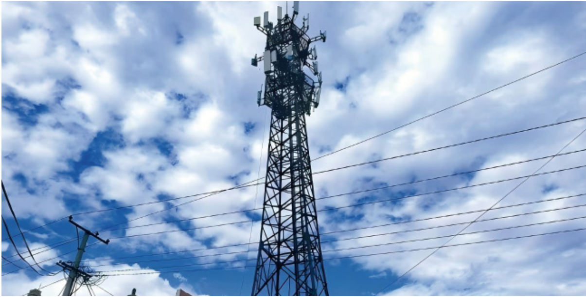
China Mobile Heilongjiang Smart Sodium Battery Project
