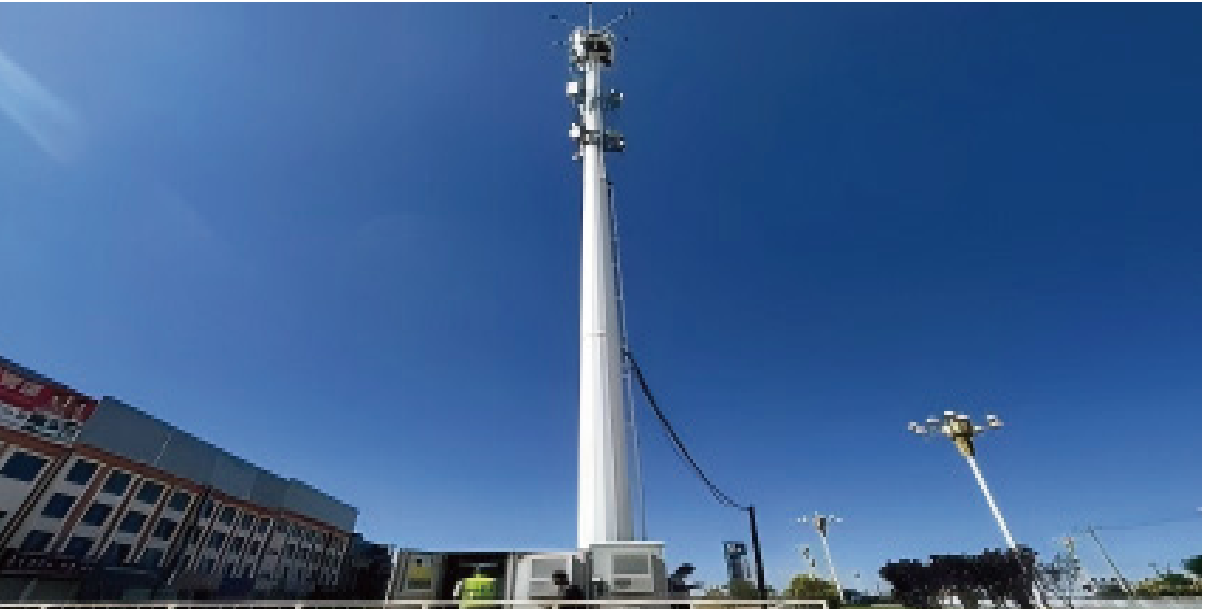
China Tower Gansu Smart Sodium Battery Project
