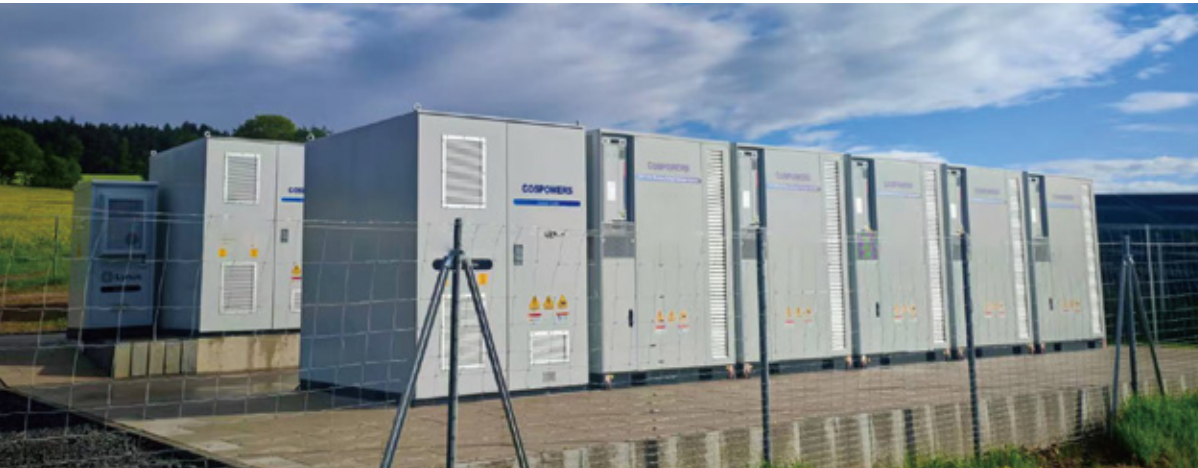
Germany 12MW/10.02MWh Energy Storage Project
