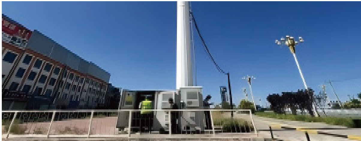
China Tower Gansu Smart Sodium Battery Project
