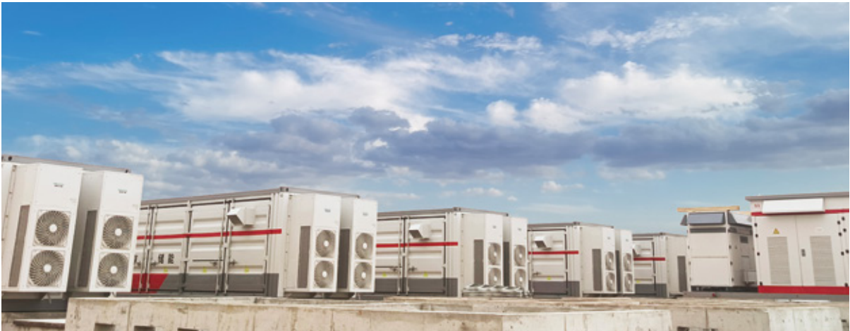
200MW/800MWh Energy Storage Project in Yinchuan, Ningxia
