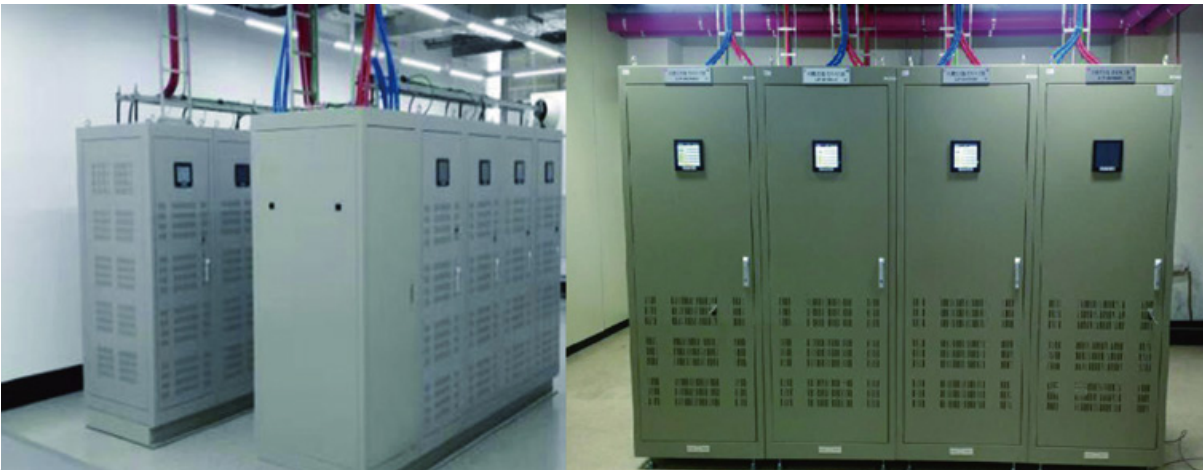
South Korea IDC Data Center Project
