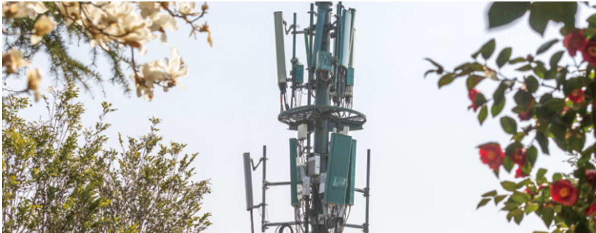
South Korea KT Telecom Base Station Project
