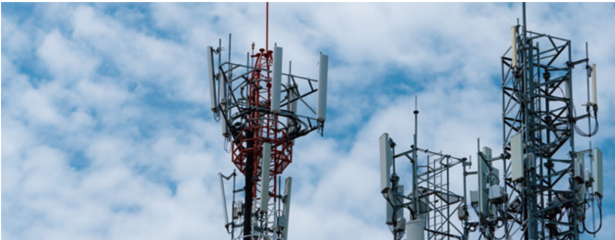
China Mobile Hunan 5G Micro-Station Integrated Project
