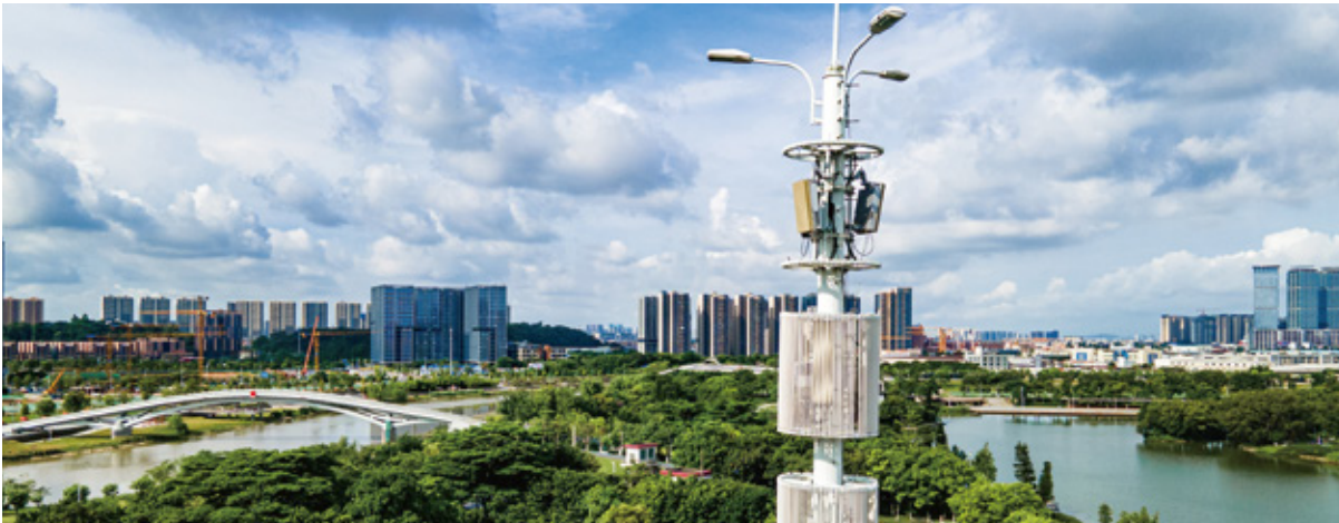
China Tower Zhejiang Smart Lithium Project
