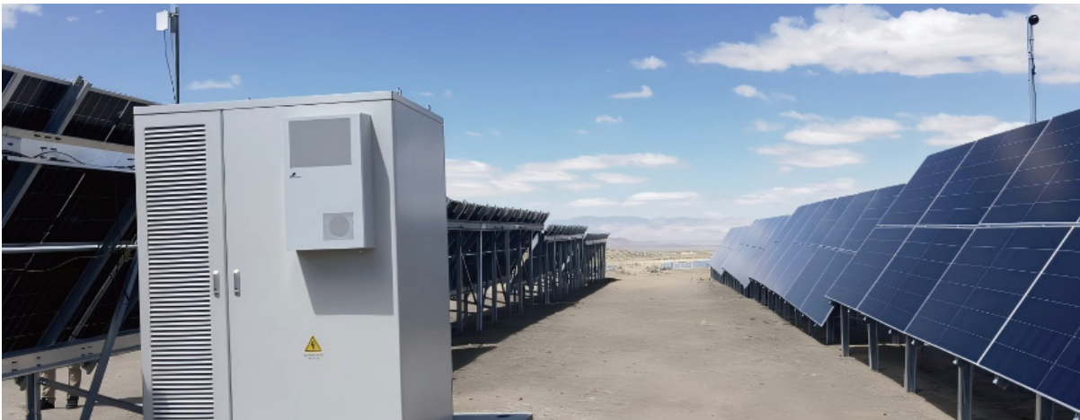
U.S. Off-Grid Solar-Storage Integrated Backup Power Project
