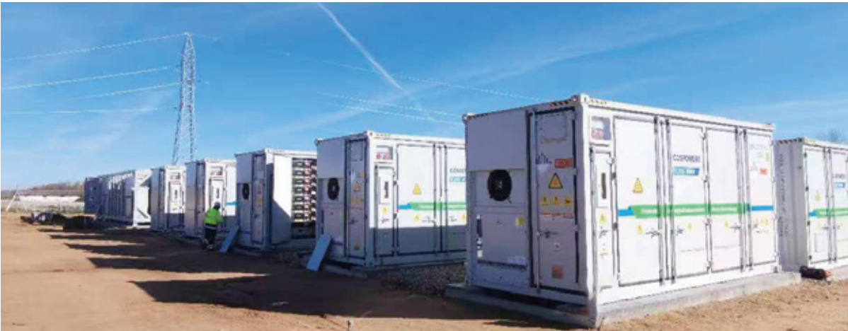
Spanish 54.92MW/250.72MWh Hybrid Energy Storage System Project
