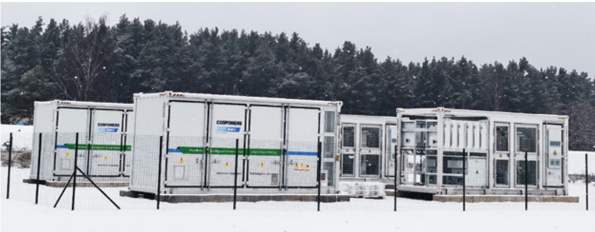
Latvia 5MW/10MWh Energy Storage System Project
