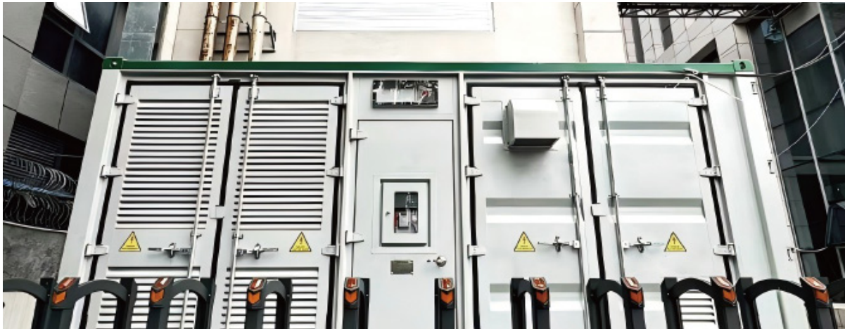
Myanmar Commercial & Industrial Energy Storage Project
