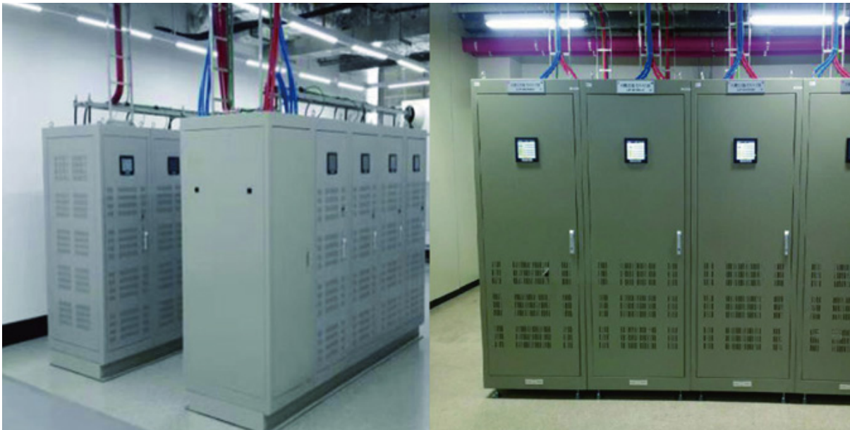
South Korea IDC Data Center Project
