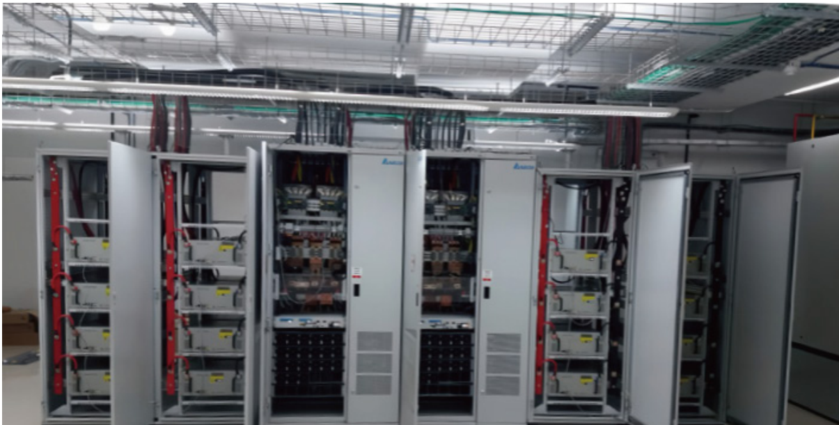
India Reliance Data Center Project
