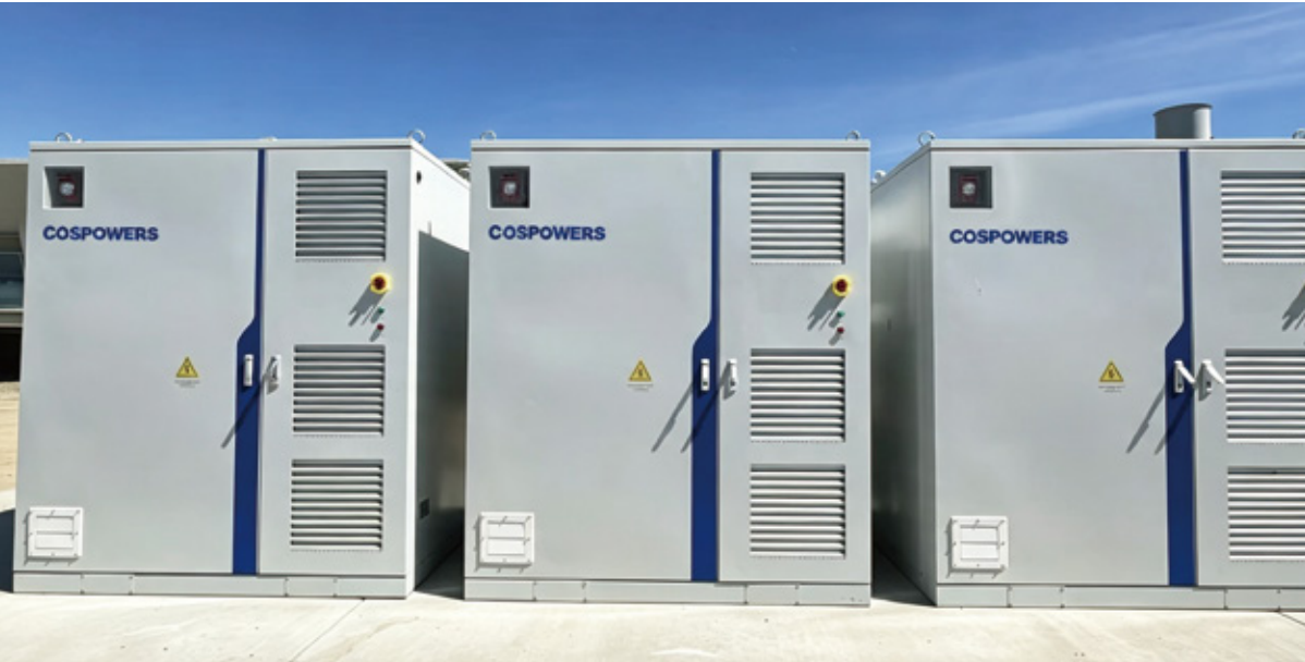
U.S. Commercial & Industrial Energy Project Time: 2025 Project Location: San Francisco, USA
