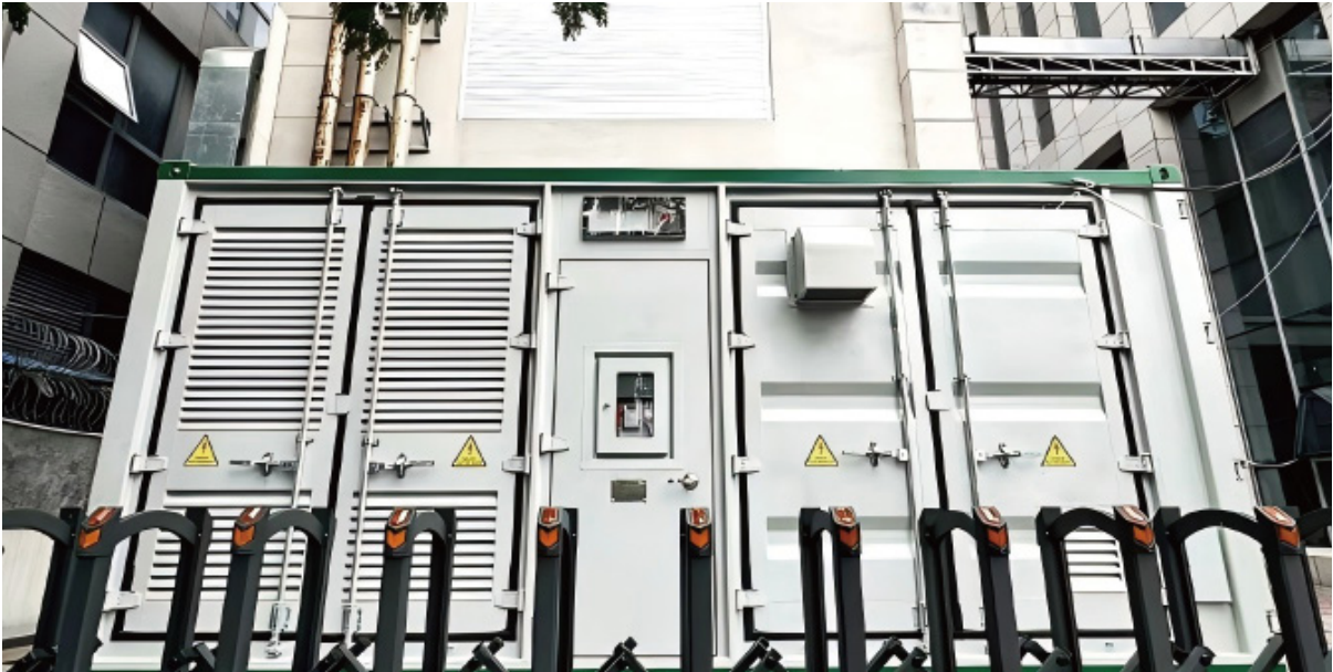
Myanmar Commercial & Industrial Energy Storage Project
