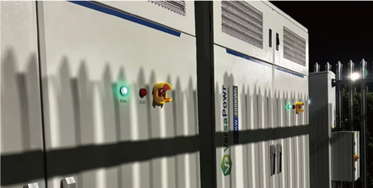
Scotland Commercial & Industrial Energy Project Time: 2025 Project Location: Glasgow, Scotland
