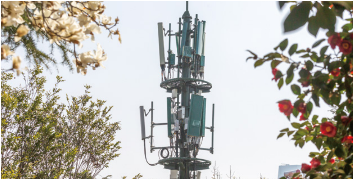
South Korea KT Telecom Base Station Project
