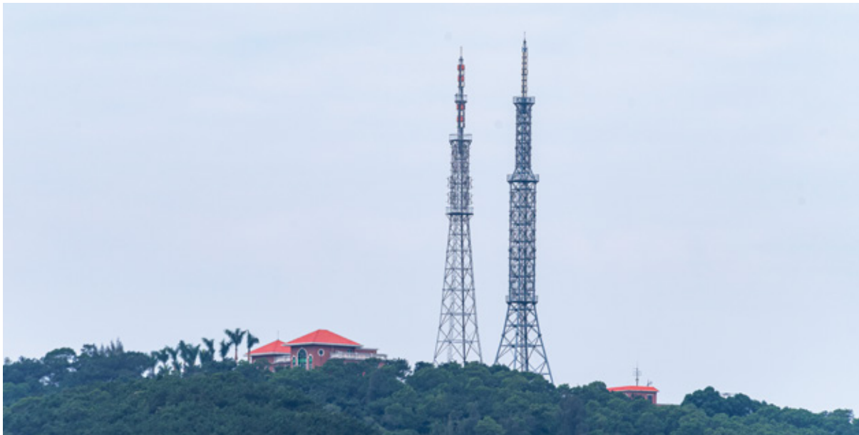
Cambodia Metfone Base Station Project
