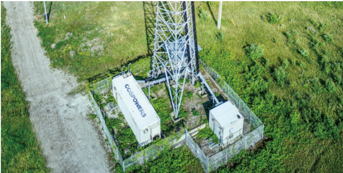
India Reliance AG3 Base Station Project
