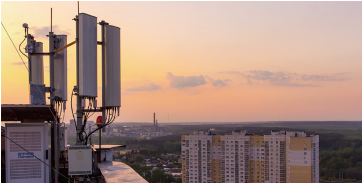
China Mobile Base Station Backup Power Project
