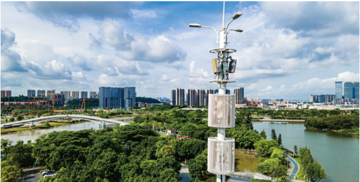
China Tower Zhejiang Smart Lithium Project
