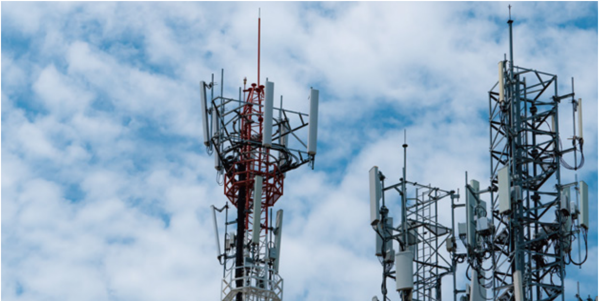
China Mobile Hunan 5G Micro-Station Integrated Project
