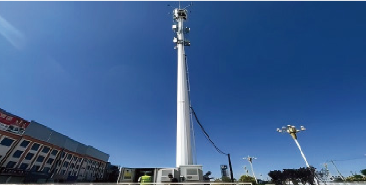
China Tower Gansu Smart Sodium Battery Project Project Time: 2024 Project Location: Tianshui,Gansu, China
