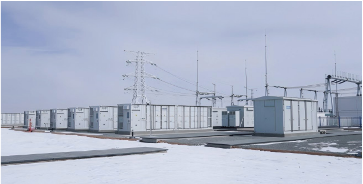
Gansu Linze 500MW Photovoltaic Desert-Control Power Generation + 40MW/80MWh Energy Storage Project Project Time: 2022 Project Location: Linze, Gansu, China Project Highlights: Flexible power control, regulating grid inflection points, smoothing power fluctuations.
