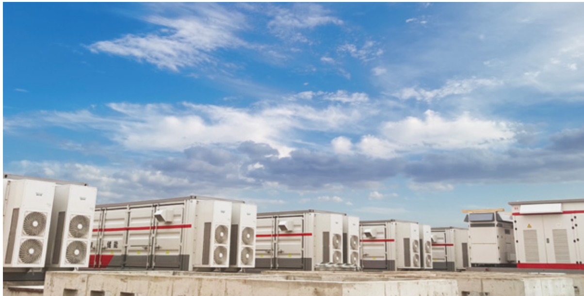
200MW/800MWh Energy Storage Project in Yinchuan, Ningxia Project Time: 2025 Project Location: Yinchuan, Ningxia Project Highlights: Innovating the sand-control economy to empower green and low-carbon development in Ningxia
