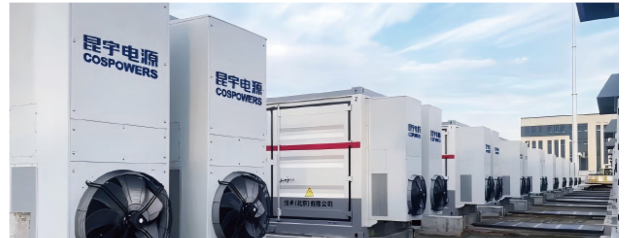
200MW Aquaculture-Photovoltaic Complementary Power Generation and 87.5MW/175MWh Energy Storage Project in Tianchang, Anhui
