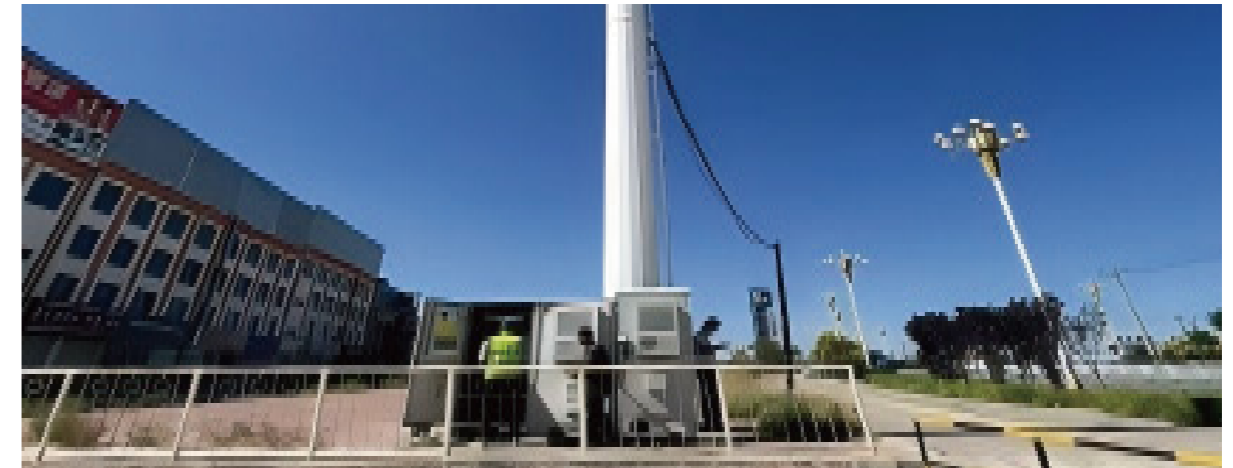
China Tower Gansu Smart Sodium Battery Project
