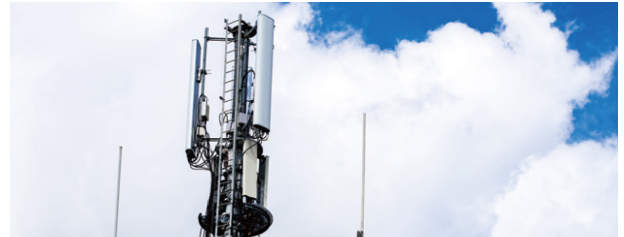
China Tower Heilongjiang Smart Sodium Battery Project
