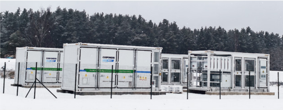
Latvia 5MW/10MWh Energy Storage System Project
