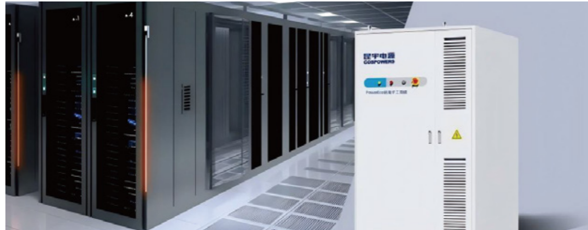
China Mobile Ningxia Data Center Distributed Photovoltaic Project
