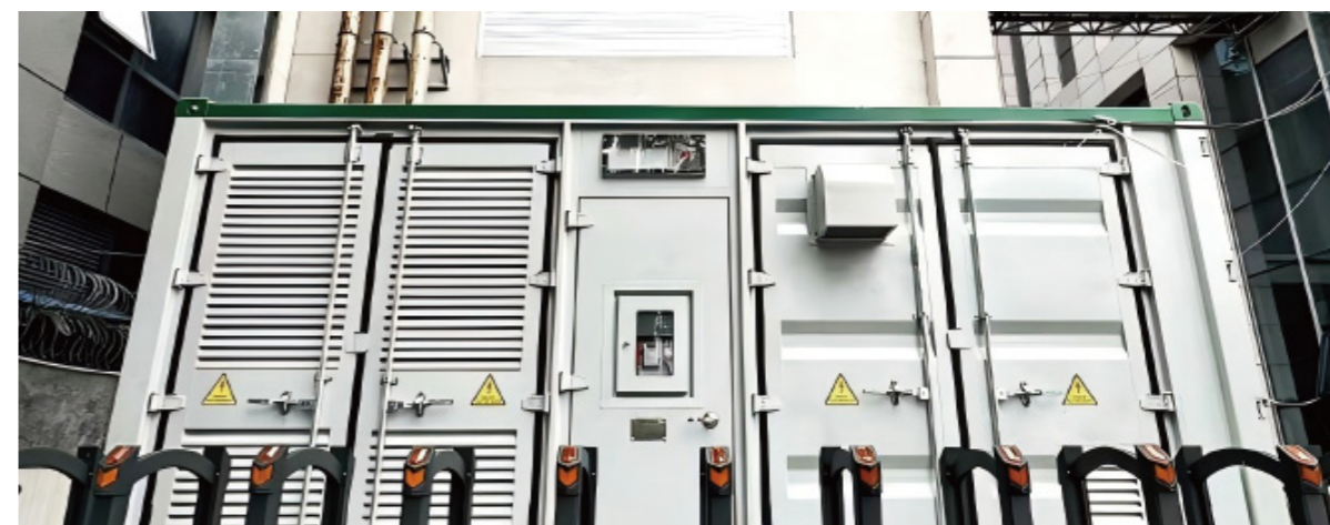
Myanmar Commercial & Industrial Energy Storage Project
