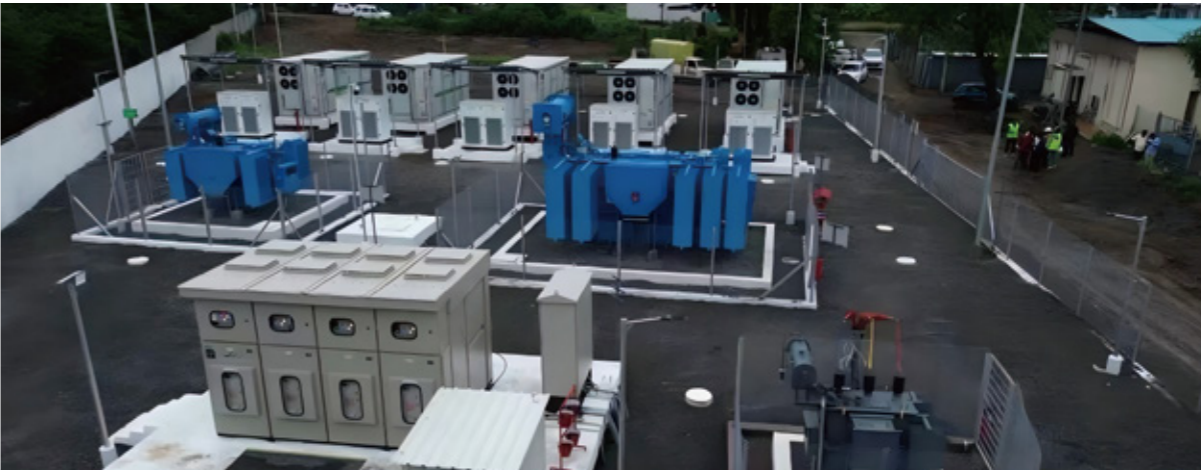
11MW/22.99MWh Energy Storage Project in India
