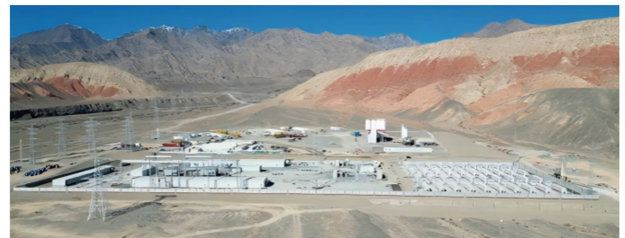
50MW Wind Power Generation and 50MW/200MWh Energy Storage Project in Wuqia, Xinjiang
