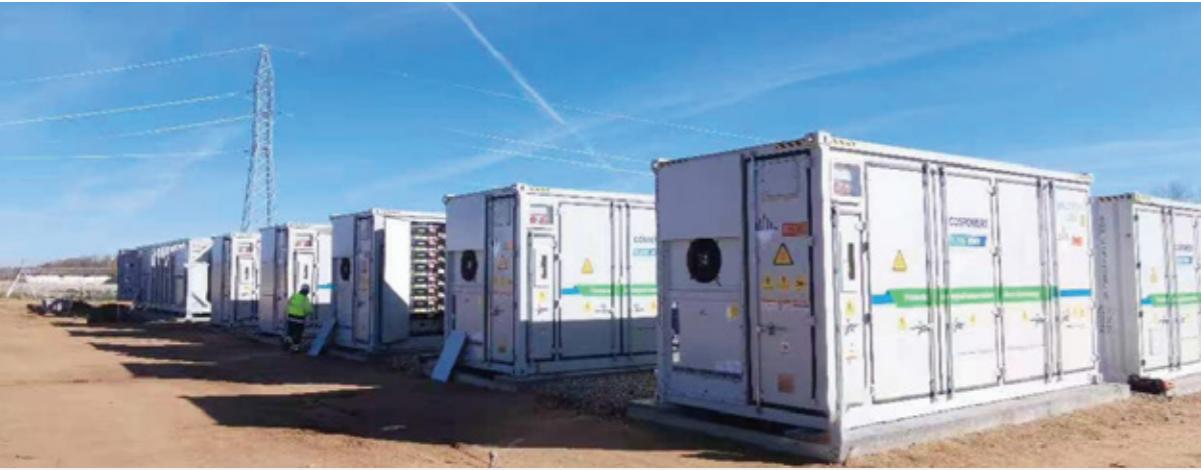
Spanish 54.92MW/250.72MWh Hybrid Energy Storage System Project
