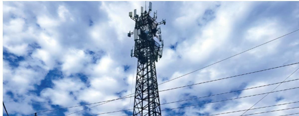
China Mobile Heilongjiang Smart Sodium Battery Project
