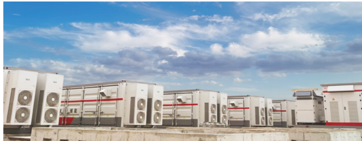
200MW/800MWh Energy Storage Project in Yinchuan, Ningxia
