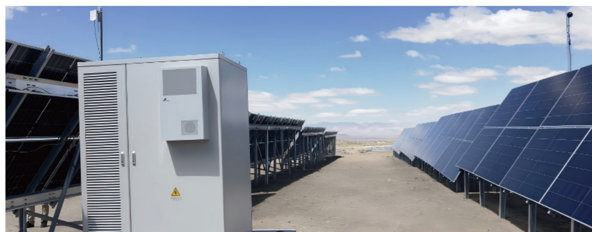
U.S. Off-Grid Solar-Storage Integrated Backup Power Project
