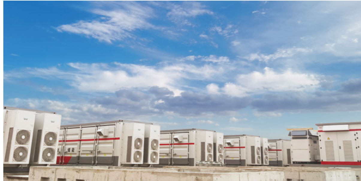
200MW/800MWh Energy Storage Project in Yinchuan, Ningxia
