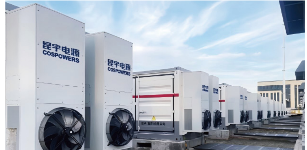
Anhui Tianchang 200MW Fishery-Photovoltaic + 87.5MW/175MWh Energy Storage Project
