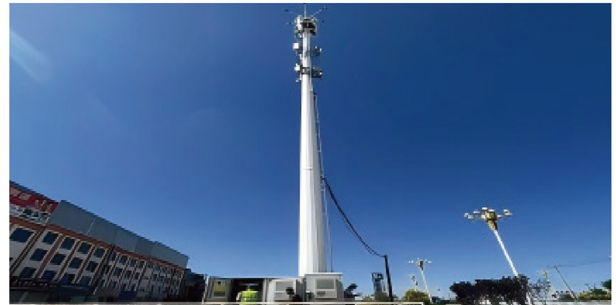
China Tower Gansu Smart Sodium Battery Project
