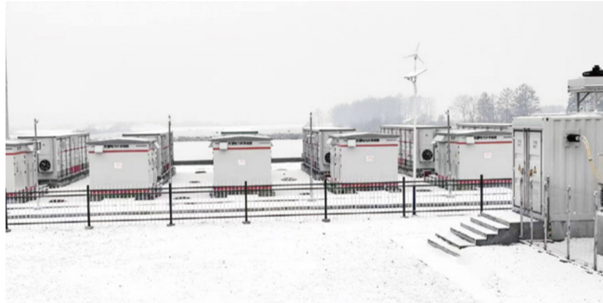
Heilongjiang Yichun Tieli Nianfeng 20MW Wind Power + 20MW/40MWh Energy Storage Project
