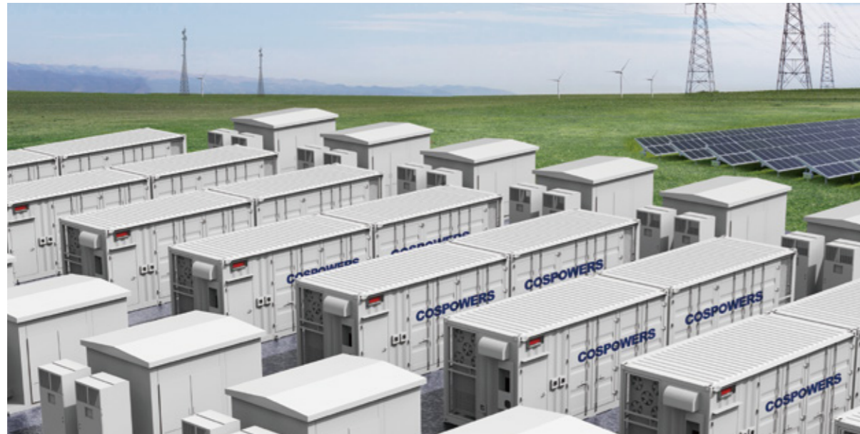
Bulgaria 200MW/800MWh Battery Energy Storage System Project Project Time: 2025 Project Location: Bulgaria Project Highlights: Ultra-large capacity, peak shaving and valley filling, supporting the European power grid.
