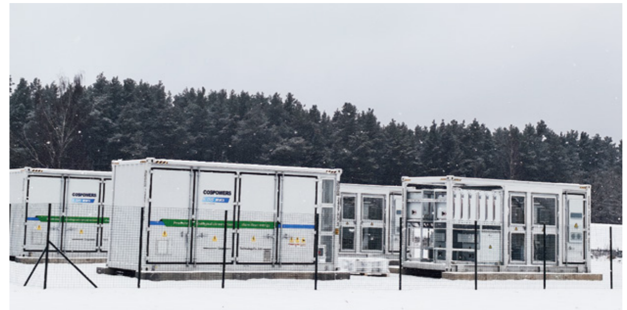
Latvia 5MW/10MWh Energy Storage System Project Project Time: 2025 Project Location: Latvia Project Highlights: Customized solution, peak shaving and valley filling, providing auxiliary grid services.
