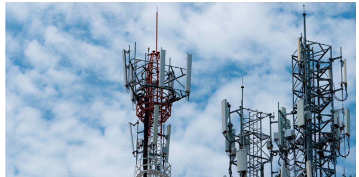
China Mobile Hunan 5G Micro-Station Integrated Project
