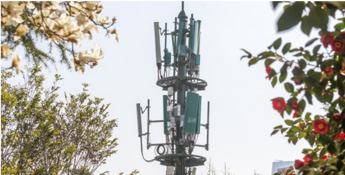
South Korea KT Telecom Base Station Project
