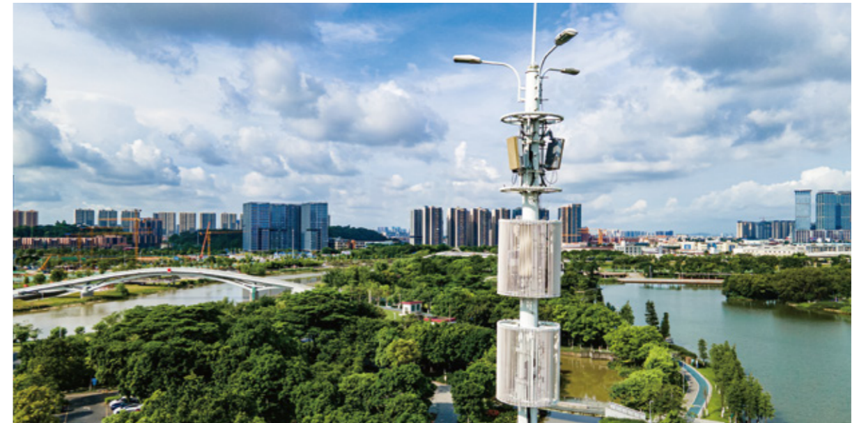
China Tower Zhejiang Smart Lithium Project
