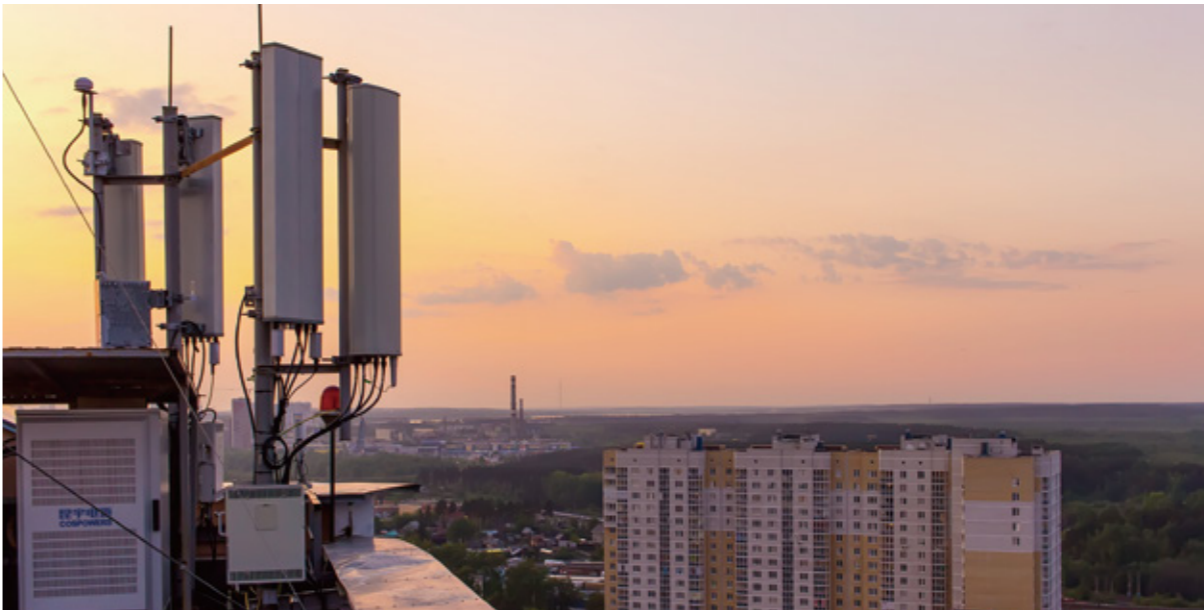
China Mobile Base Station Backup Power Project
