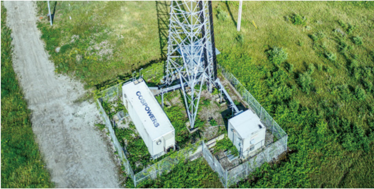
India Reliance AG3 Base Station Project
