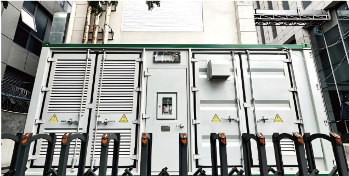
Myanmar Commercial & Industrial Energy Storage Project Project Time: 2024 Project Location: Myanmar
