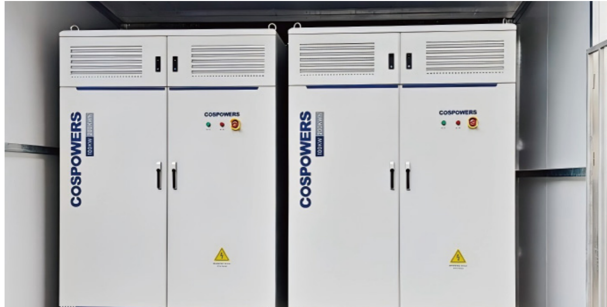
Shenzhen Pinghu Peak Shaving & Valley Filling Commercial & Industrial Energy Storage Project
