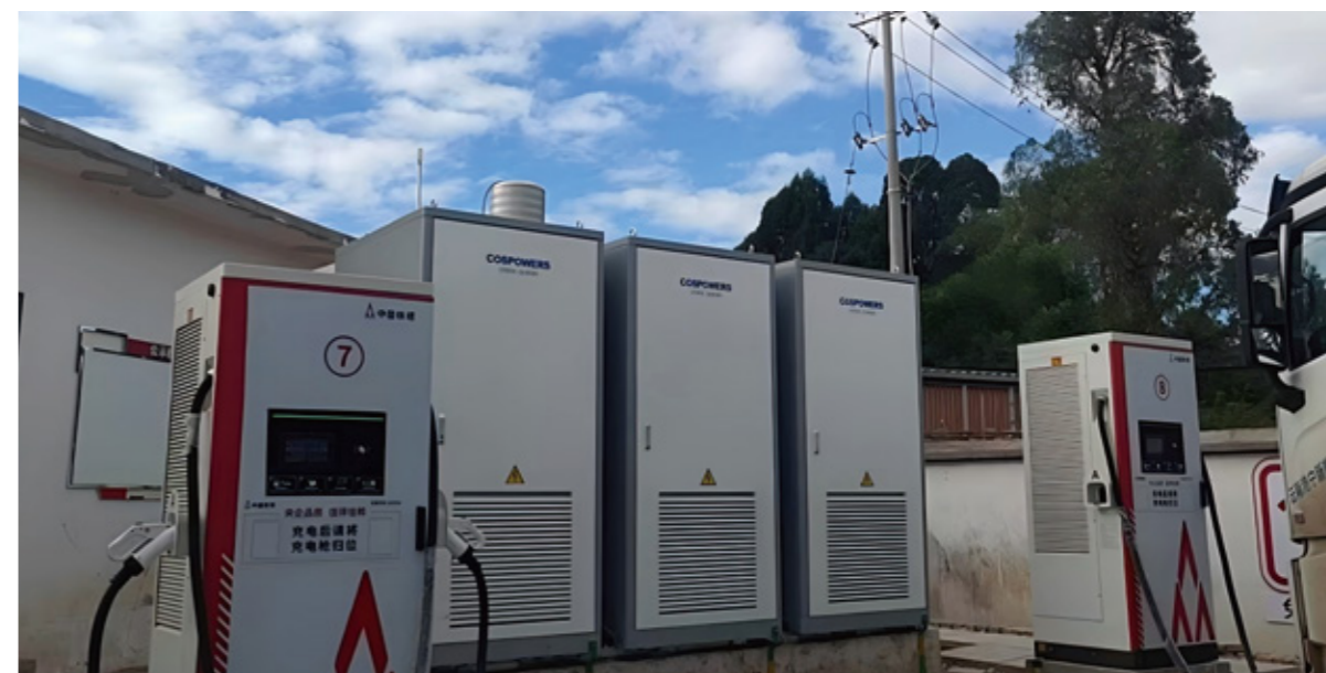
Kunming Shilin Beida Village Heavy-Duty Truck Charging Station Energy Storage Project
