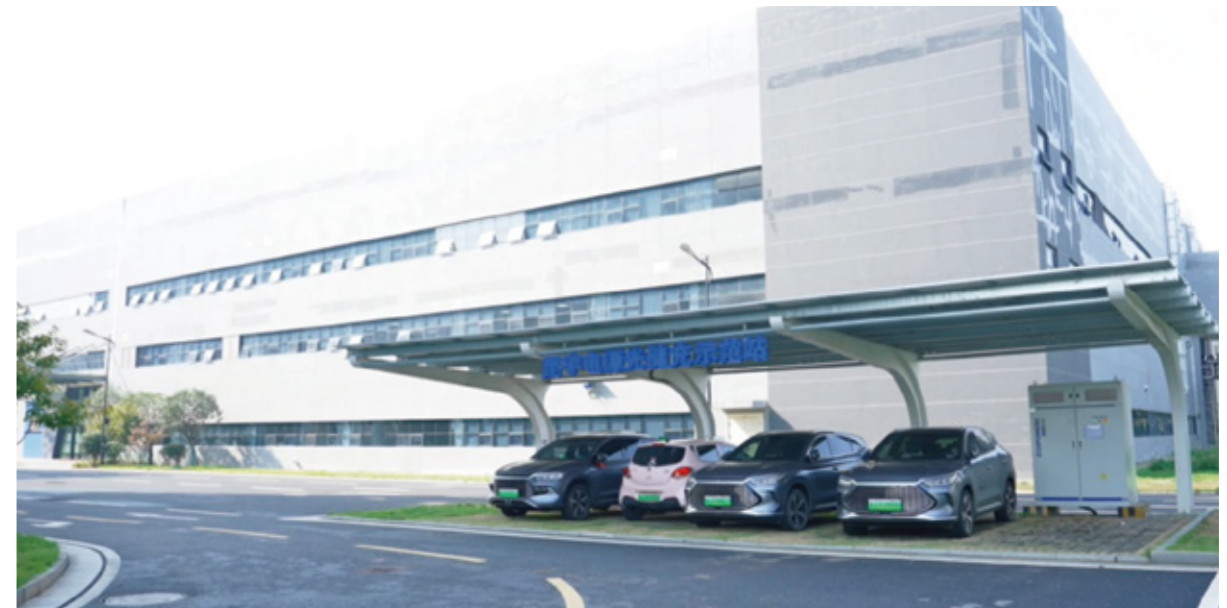
Hunan Changde Solar-Storage-Charging Integrated Station Commercial & Industrial Energy Storage Project
