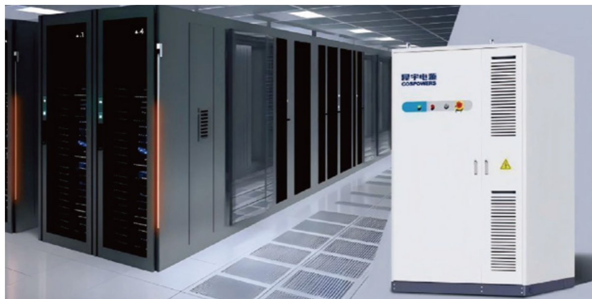
China Mobile Ningxia Company Data Center Distributed Photovoltaic Project
