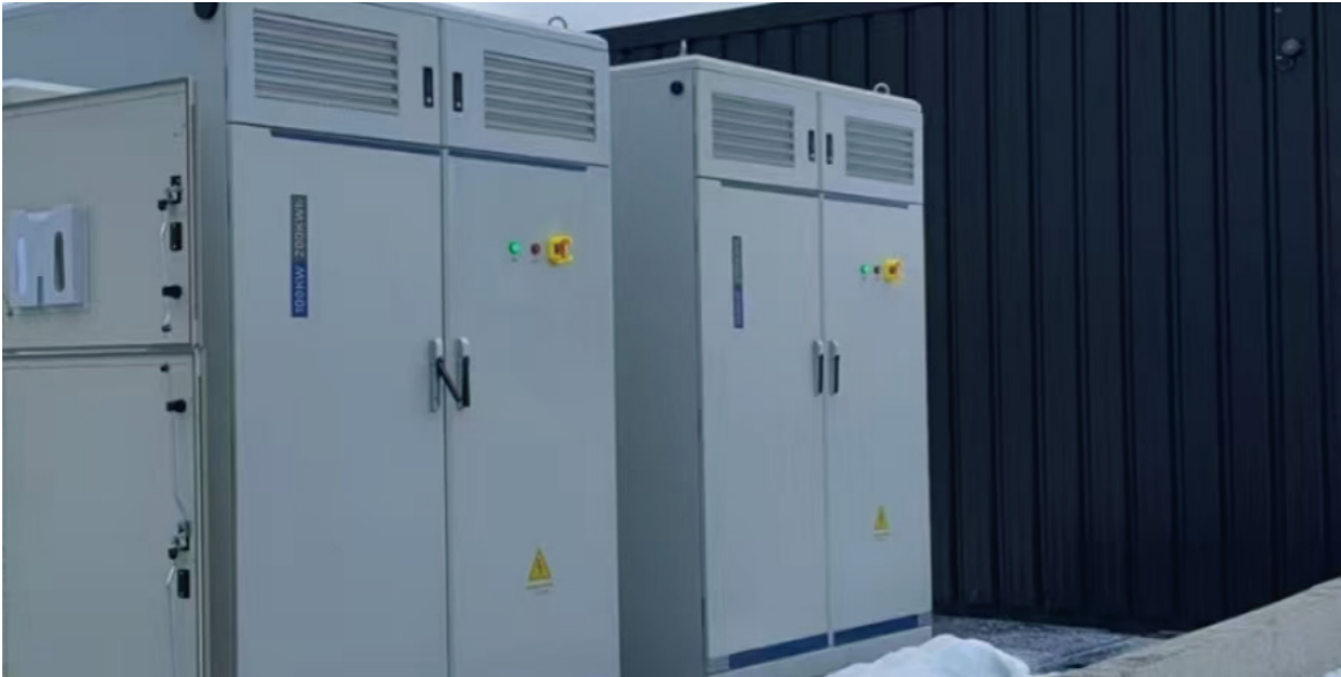
Norway Commercial & Industrial Energy Project Time: 2024 Project Location: Norway
