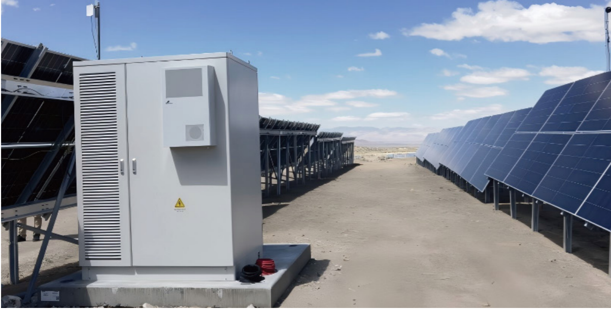
U.S. Off-Grid Solar-Storage Integrated Backup Power Project Project Time: 2024 Project Location: United States
