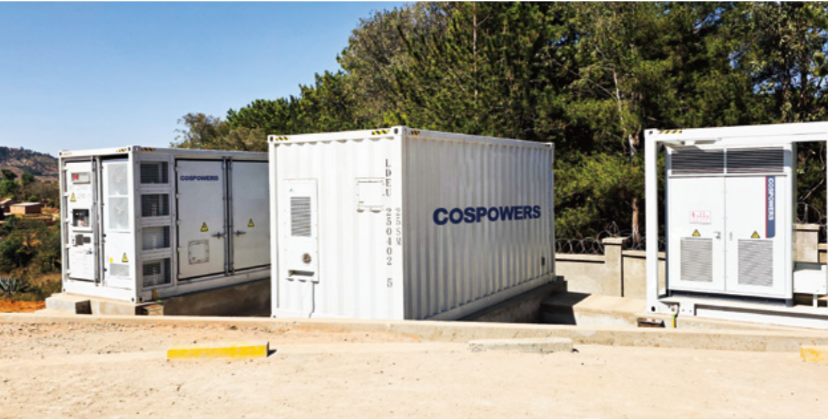
Madagascar IVATO Industrial Park Integrated Photovoltaic-Energy Storage-Diesel Smart Microgrid Project
