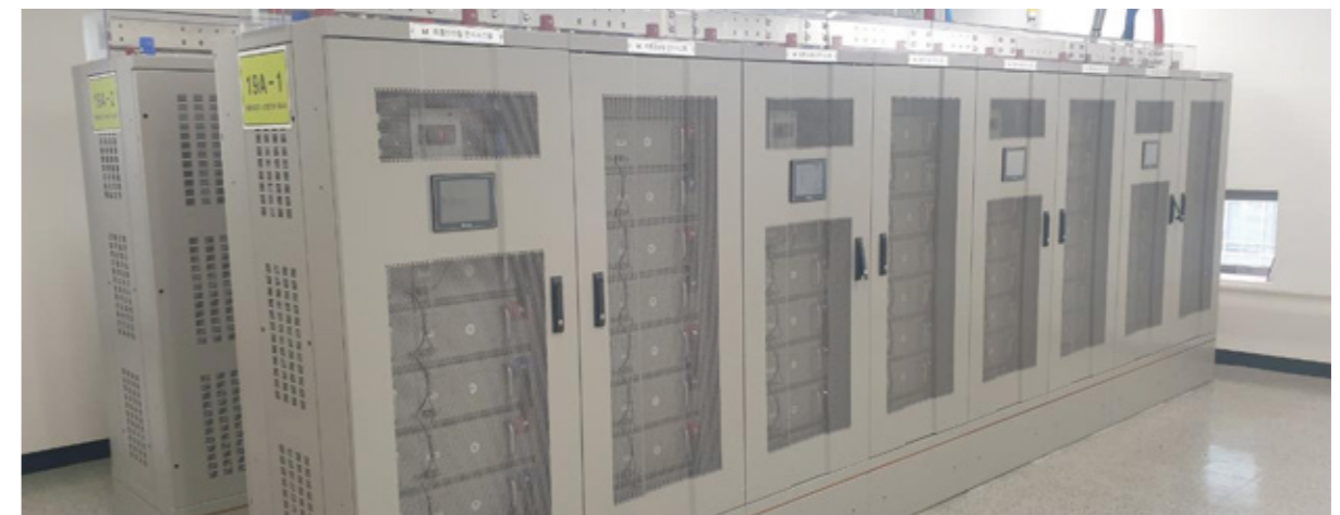
South Korea Cheongju Data Center UPS Backup Lithium
