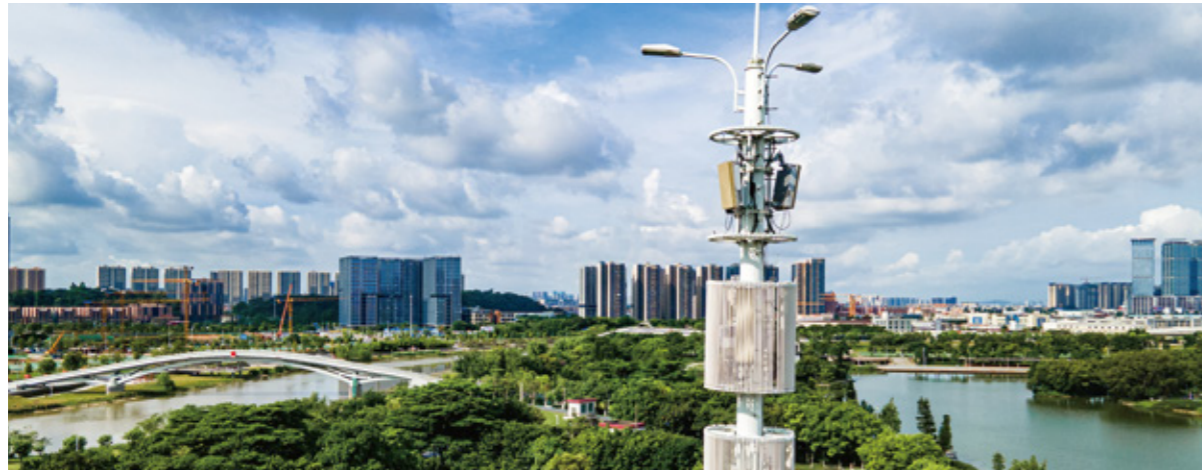
China Tower Zhejiang Smart Lithium Project
