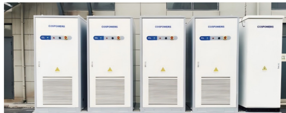
Jiangsu Taixing Garment Washing Factory Commercial & Industrial Energy Storage Project
