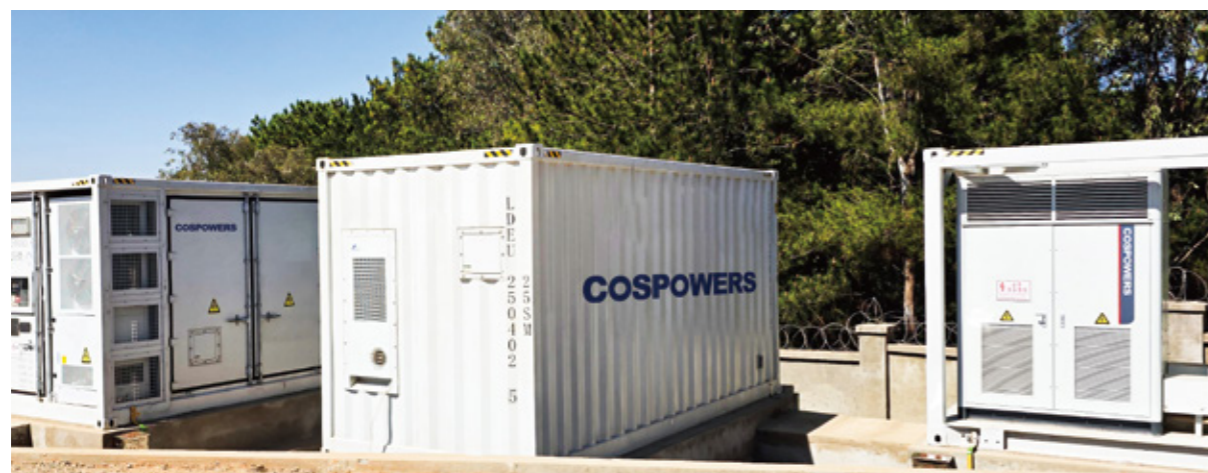
Madagascar IVATO Industrial Park Integrated Solar-Storage-Diesel Smart Microgrid Project
