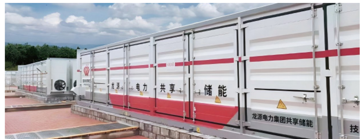
80MW/160MWh Wind Power Energy Storage Project in Weining, Guizhou
