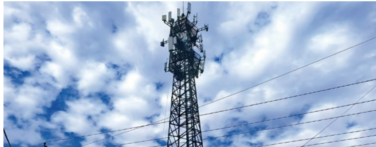
China Mobile Heilongjiang Smart Sodium Battery Project
