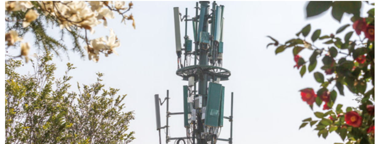
South Korea KT Telecom Base Station Project
