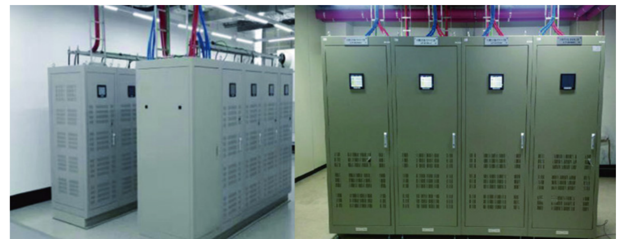
South Korea IDC Data Center Project
