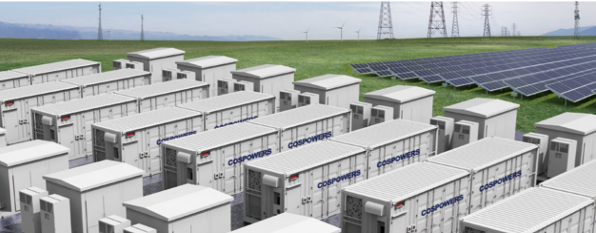
Bulgaria 200MW/800MWh Battery Energy Storage System (BESS) Project
