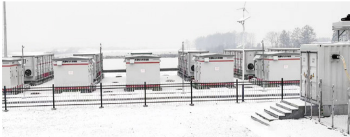
20MW Wind Power and 20MW/40MWh Battery Energy Storage Project in Nianfeng, Tieli, Yichun, Heilongjiang
