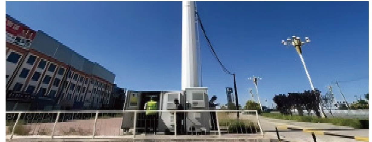
China Tower Gansu Smart Sodium Battery Project
