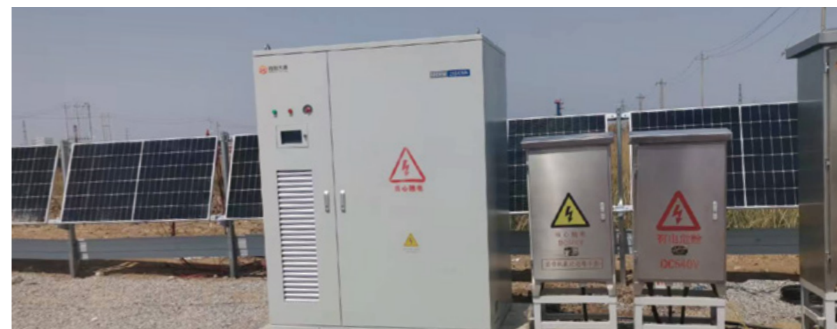
Shandong Oilfield DC Microgrid with Flexible Solar-Storage-Wind Integrated Energy Storage System
