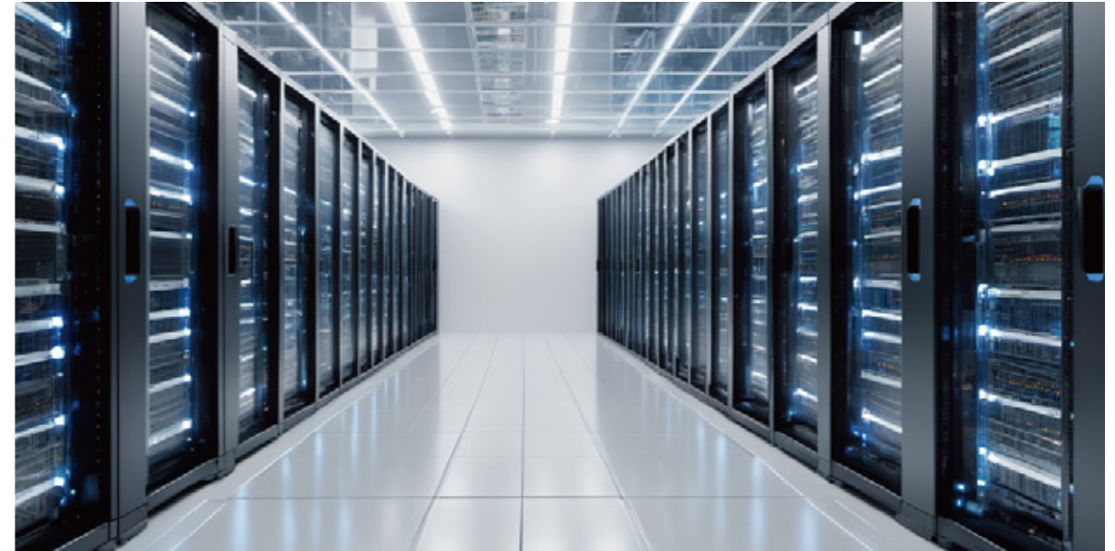
China Unicom Shanxi Data Center Project
