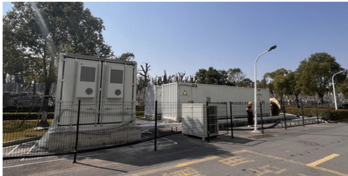
Shanghai Mobile Lingang IDC Data Center UPS Project
