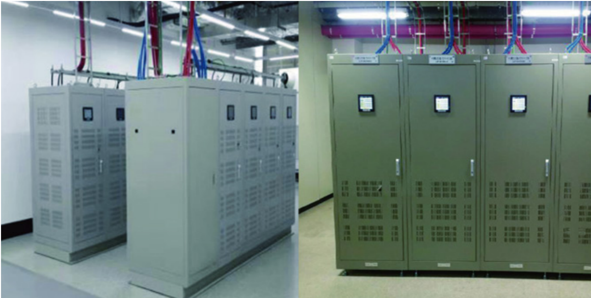
South Korea IDC Data Center Project
