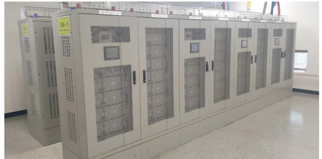
South Korea Cheongju Data Center UPS Backup Lithium Batteries
