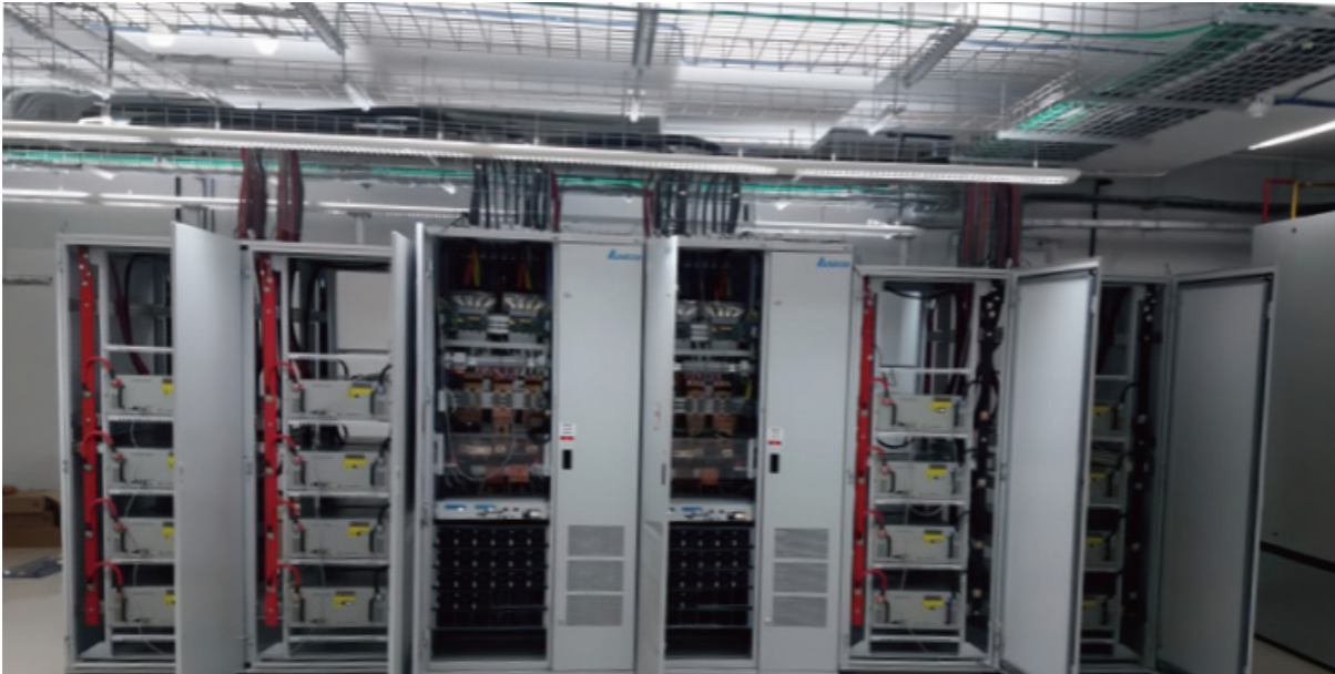
India Reliance Data Center Project
